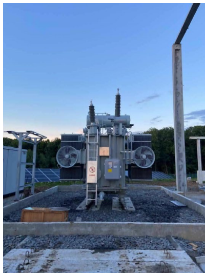
SFZ11-25000/115 Ukraine Substation
