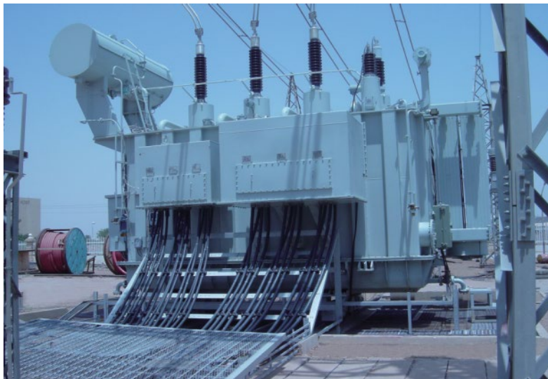
SFSZ11-60000/132 Sudan Showak Substation
