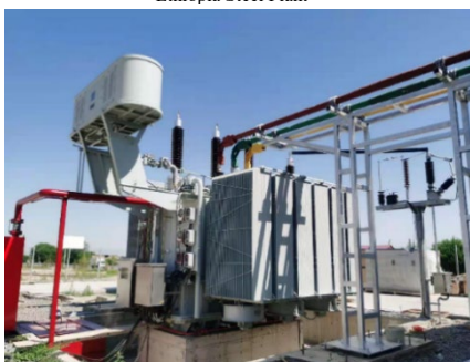
SFZ11-63000/110 Uzbekistan Samarkand Steel Works
