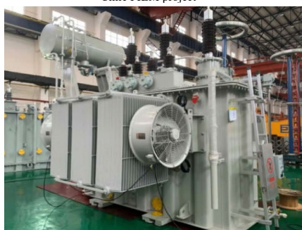
SF-24000/66 Ecuador Substation
