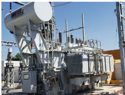
SFZ-20000/66 Chile San Gregorio Substation
