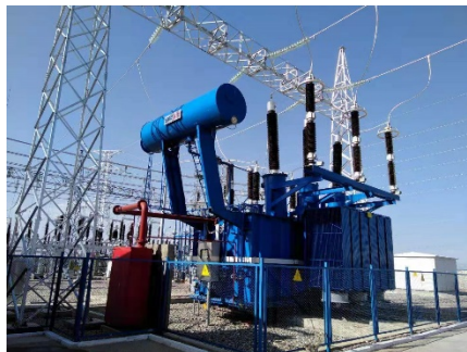
OSSFZ-125000/230 Kyrgyzstan Talas 220kV Substation
