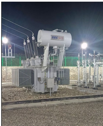
SZ-6300/110 Tajikistan Qozideh Substation
