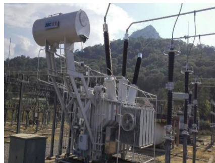
SF-25000/110 Albania Substation
