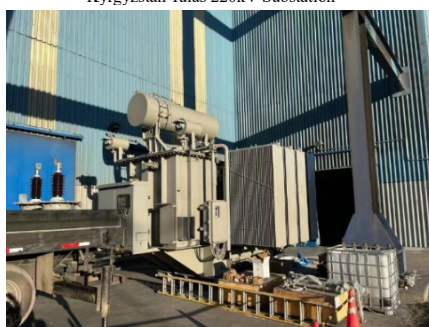
SFFZ-60000/20 Chile PIEM project
