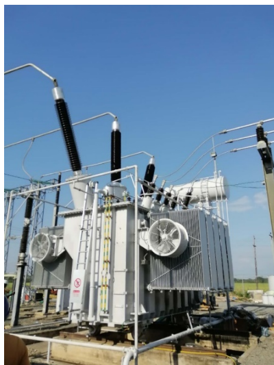
SFZ-45000/220 Tanzania KITADU Substation
