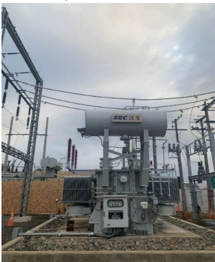
SFZ-30000/66 Chile Longavi Substation
