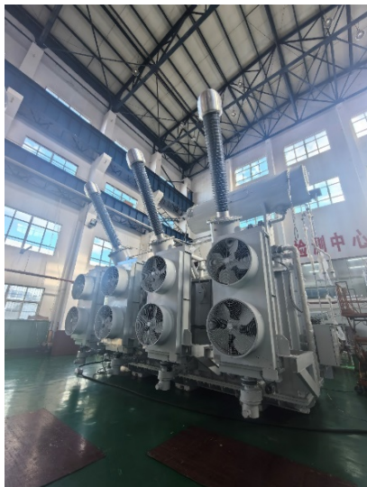
SFFPZ-160000/220 Russia Substation
